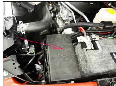
-unclip a fuse box
